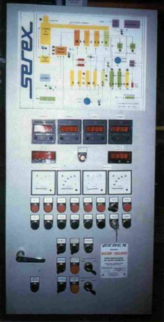
PAINEL DE CONTROLE
