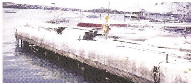
Pier no Royal Bermuda Yacht Club e Central de energia de Tynes Bay, Bermudas
